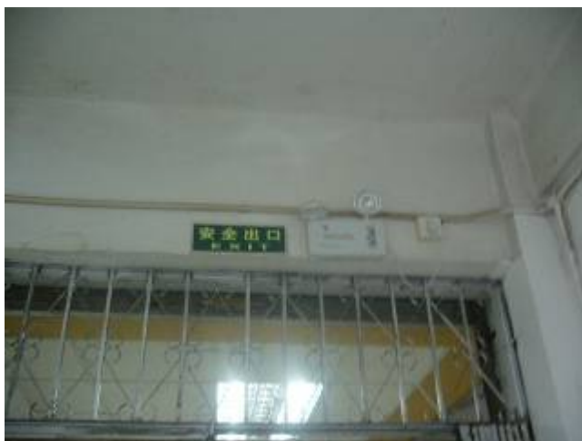
1. evacuation exit lighting
