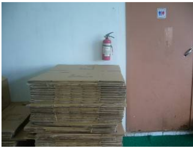
3. Extinguisher in factory: Found 1pc per emplacement and blocked.
