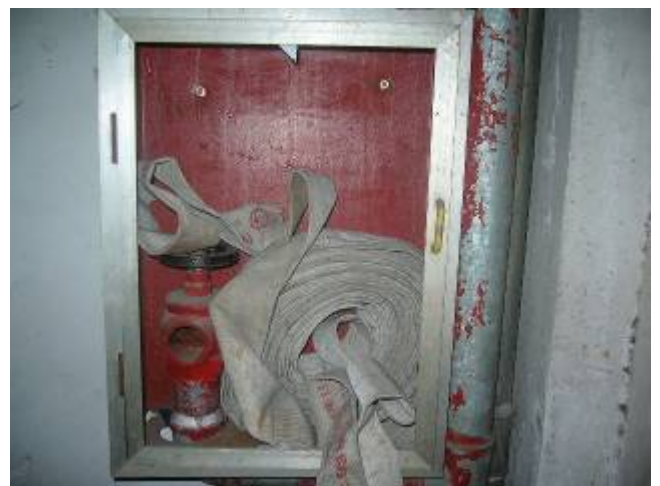
2. Fire hoses in Factory: found 1pc malfunction.
